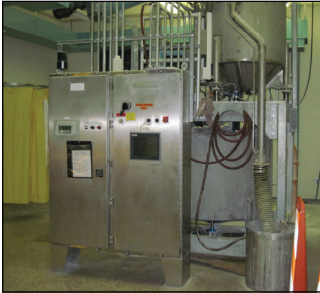
Lime Slaking System at LCWTP
